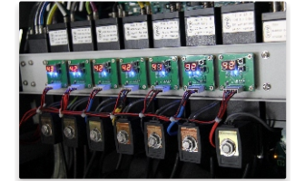
Negative Pressure System
