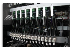
Negative Pressure System
