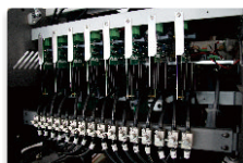
Negative Pressure System
